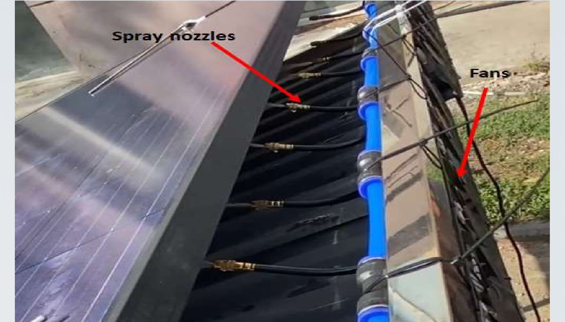
Fig.4. PV panel cooling system
