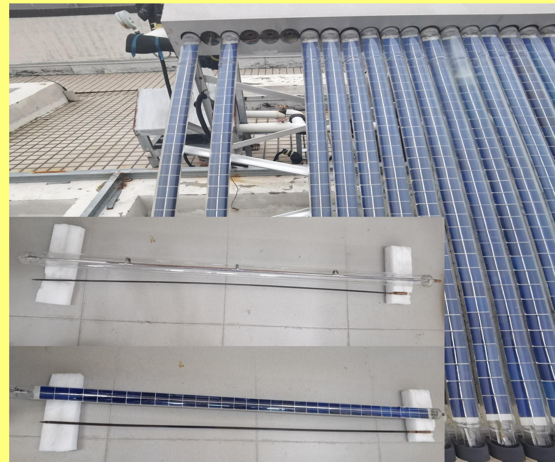
Fig. 2. Practical vacuum tube PV/T system.
